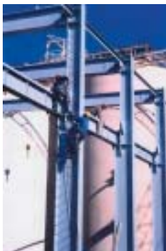
30.000 sq. m of steel construction protected at the Arauco II plant in Chile.
